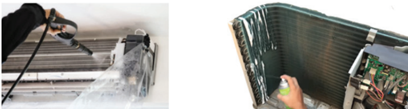
Figure 4.1: Cleaning of Condenser & Evaporator Coil
